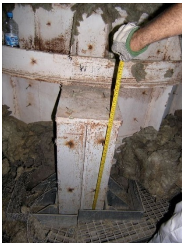
Figure 4. Chimney hanger support s
