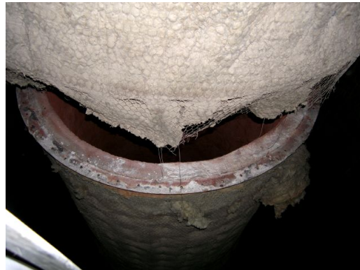
Figure 13. chimney spool fall
