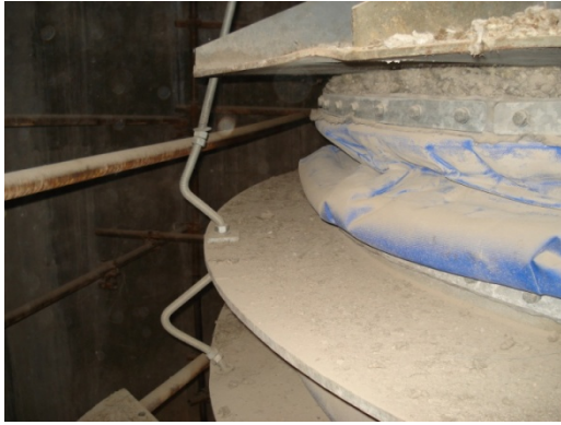
Figure 8. Damaged expansion joint
