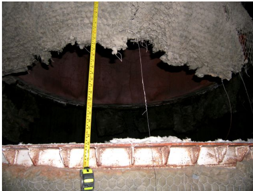
Figure 12. chimney spool fall
