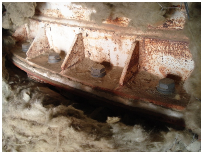
Figure 5.spools flange with stud bolt
